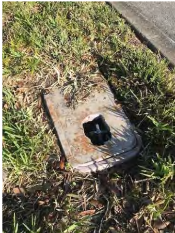
Villa sol CDD Valve box
