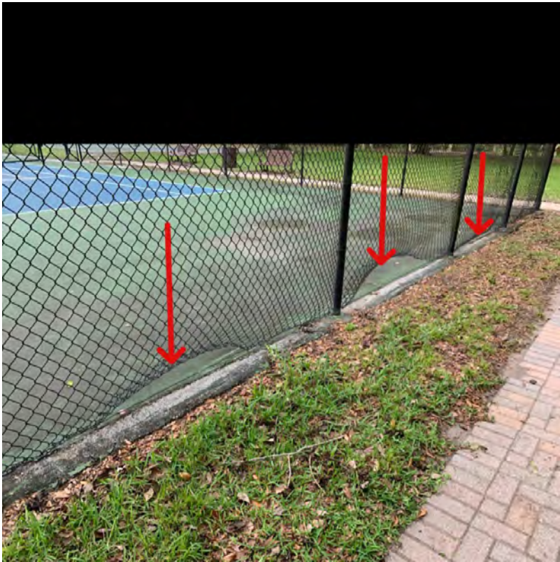
Item 3 Assigned To Inframark Repair open gaps in the tennis court fence.
