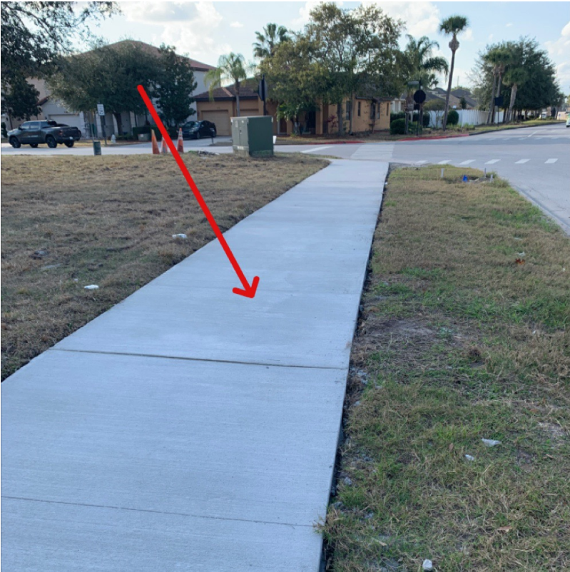
Item 6 Assigned To ToHo Water Contractors Sidewalk replacement is completed at the Puerta de Sol Blvd.
