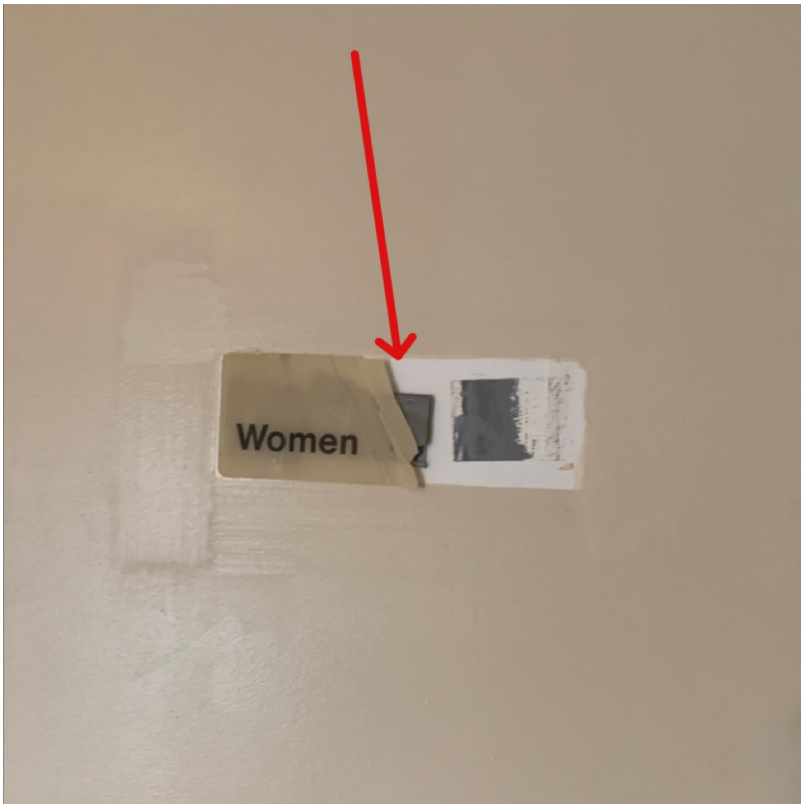
Item 2 Assigned To Inframark Replace broken female gender identification sign.
