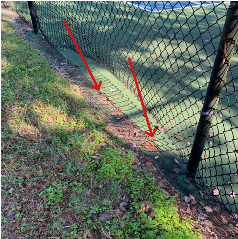
Item 6 Assigned To Inframark (Club Attendant) Repair chain link fence around the Tennis Court.
